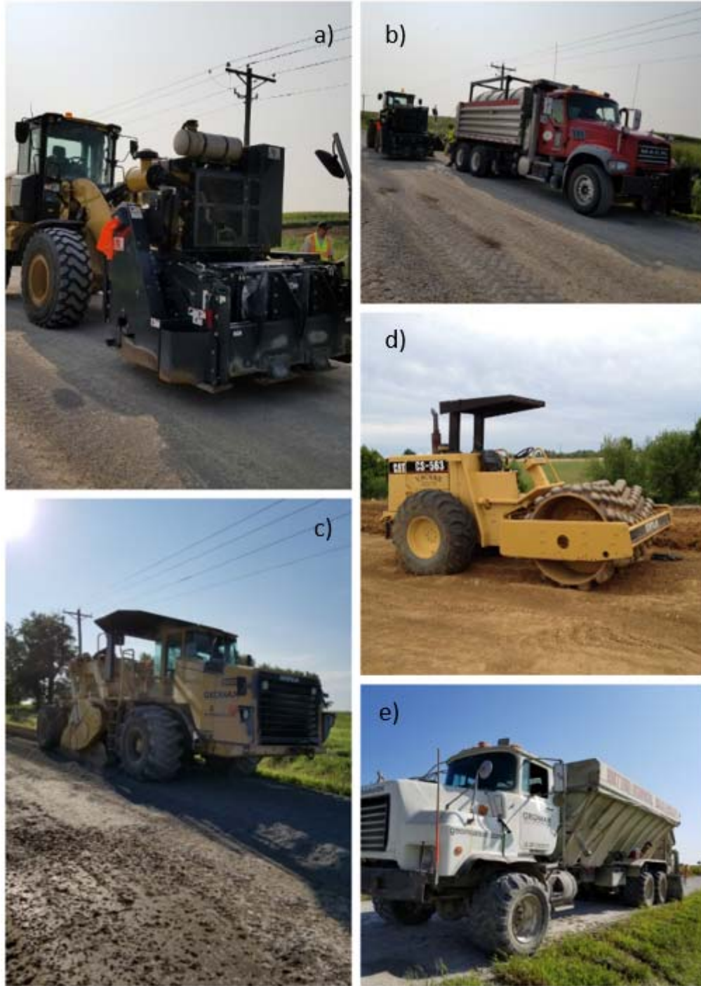
Figure 25 Equipment used for chemically stabilized sections a) RoadHog reclaimer b) water truck with chemical stabilizer added to tank connected to RoadHog c) road reclaimer d) sheepfoot vibratory compactor e) powder spreader truck
